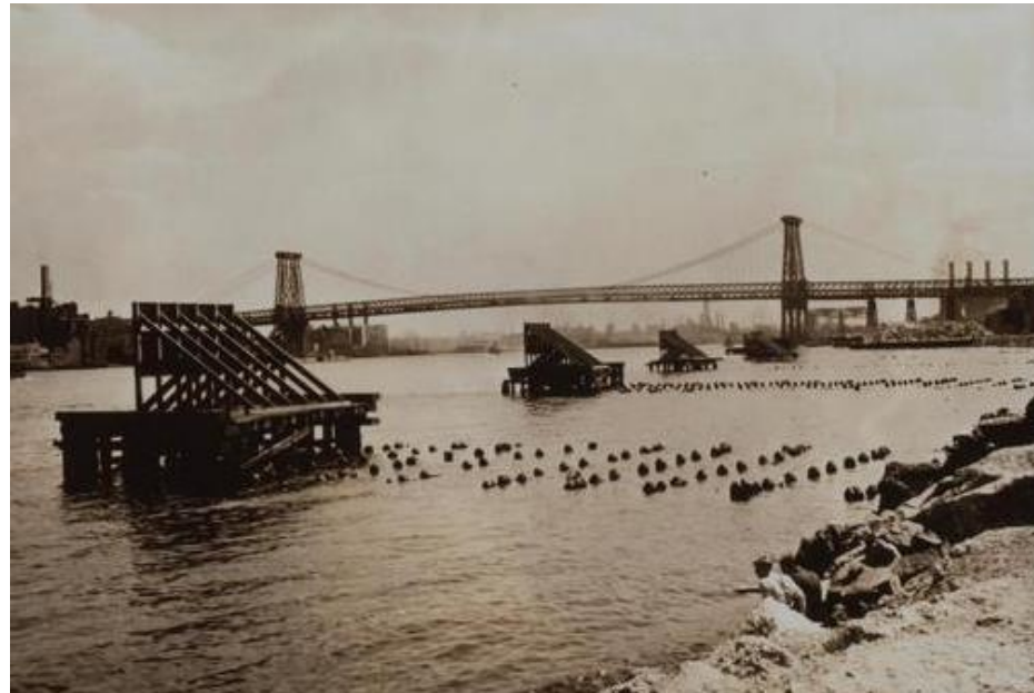
Bulkheads and pier stumps during demolition for East River Park and East River Drive – 1937
