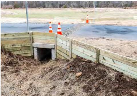
Small Mammal / Herp Underpass
